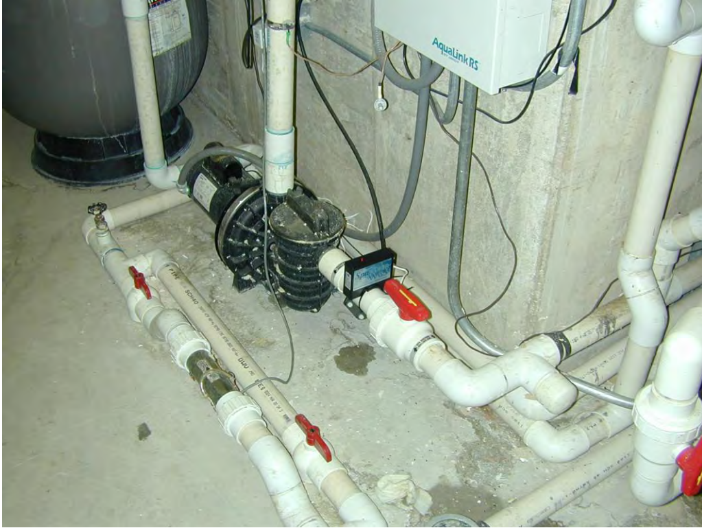
Photograph of installed HydroFLOW water conditioner
